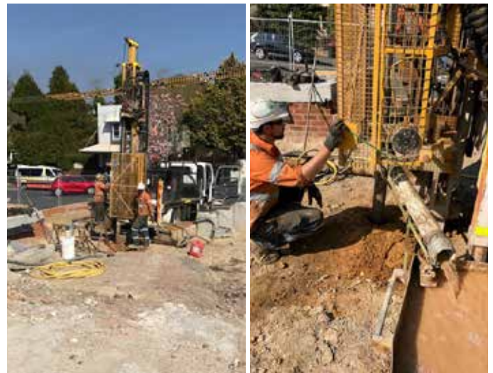
Preparations for the new club began with soil samples being taken on the site
